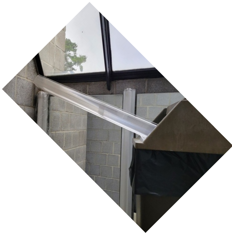
Light lens channeling water drips into a trash can.
