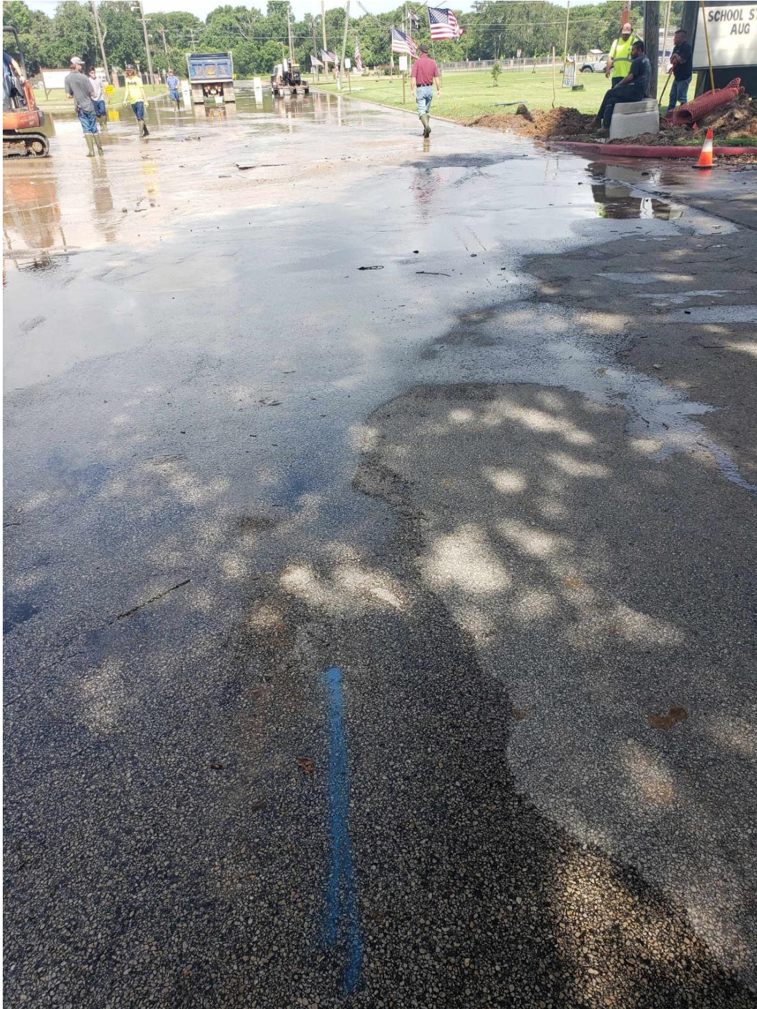
Water line break on Grand Ave. in September caused by Boring Contractor who paid for the repairs
