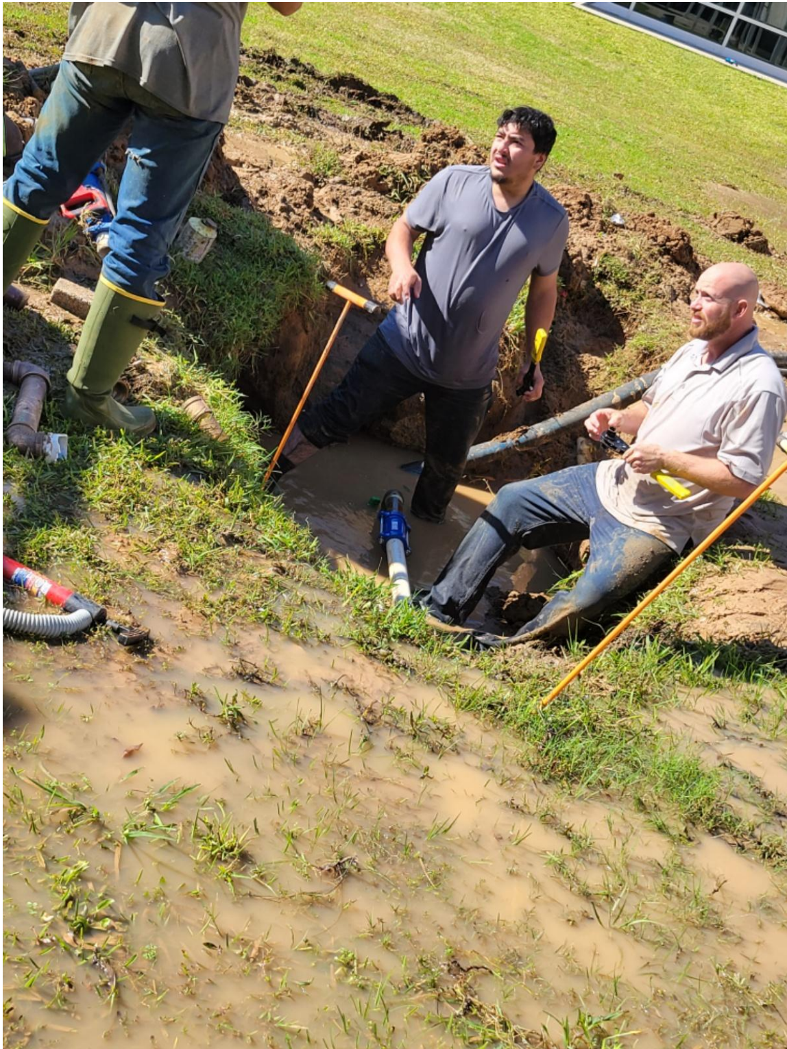
Water leak at Liberty High School; Dale Pitts and Stephen Davila
