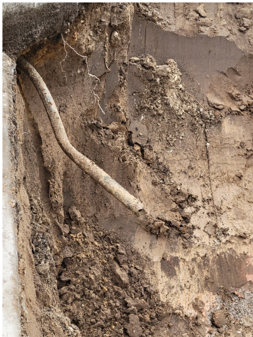
No more sinkhole!
