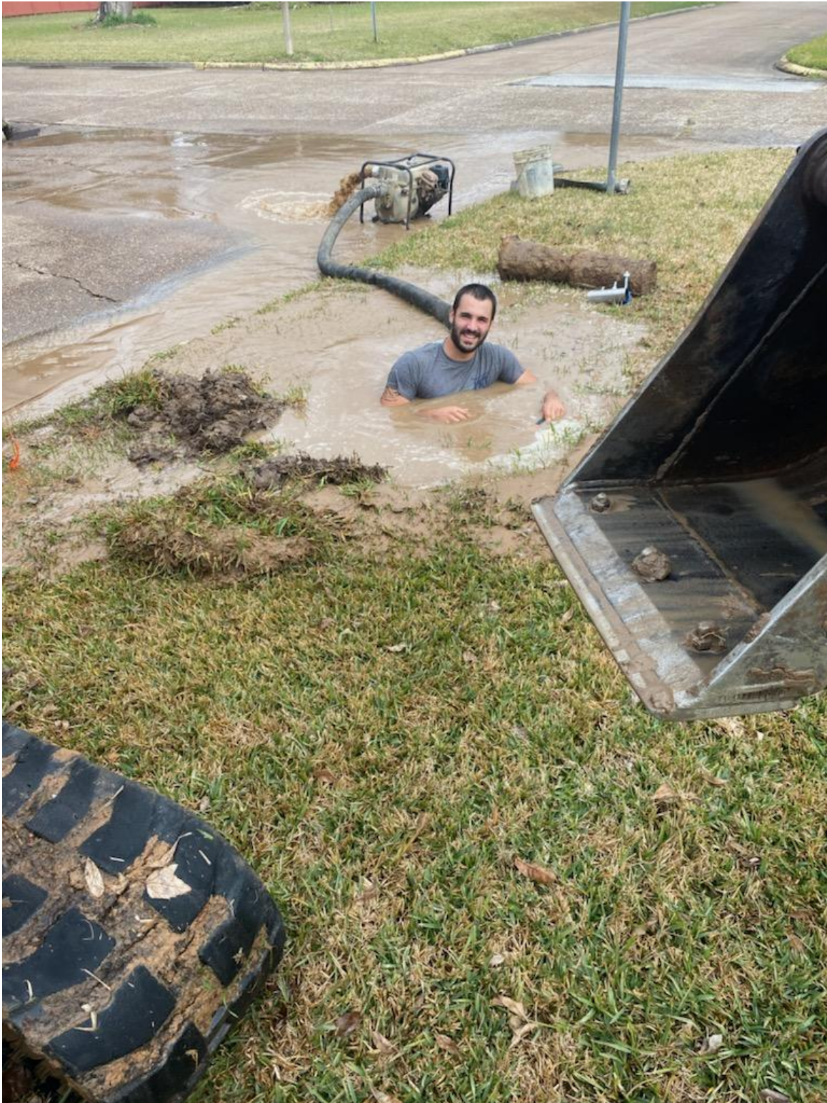
Water leak at 1622 Cos St.; Christian Ecker
