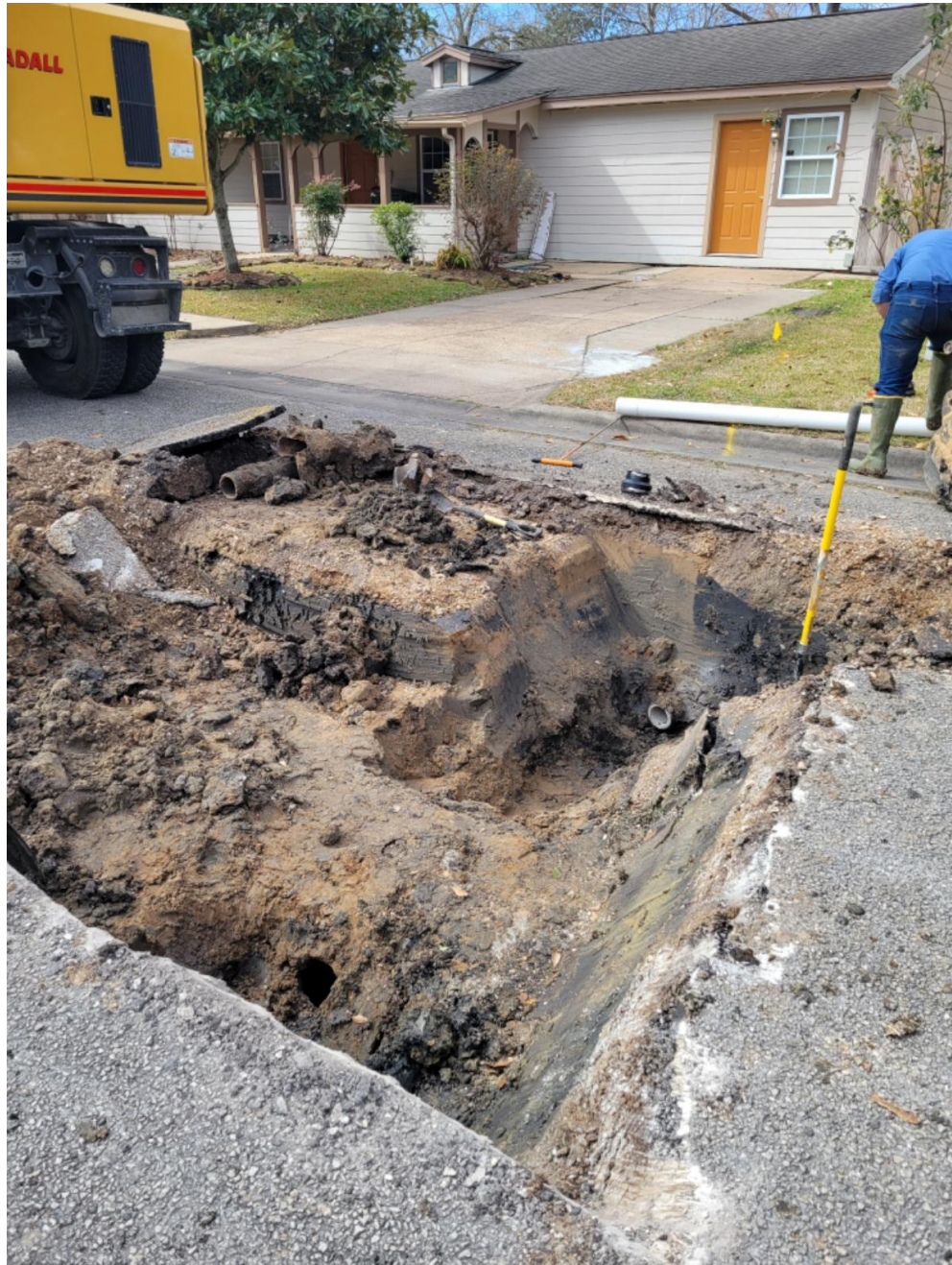
Storm drainage cavity on Woods St.
