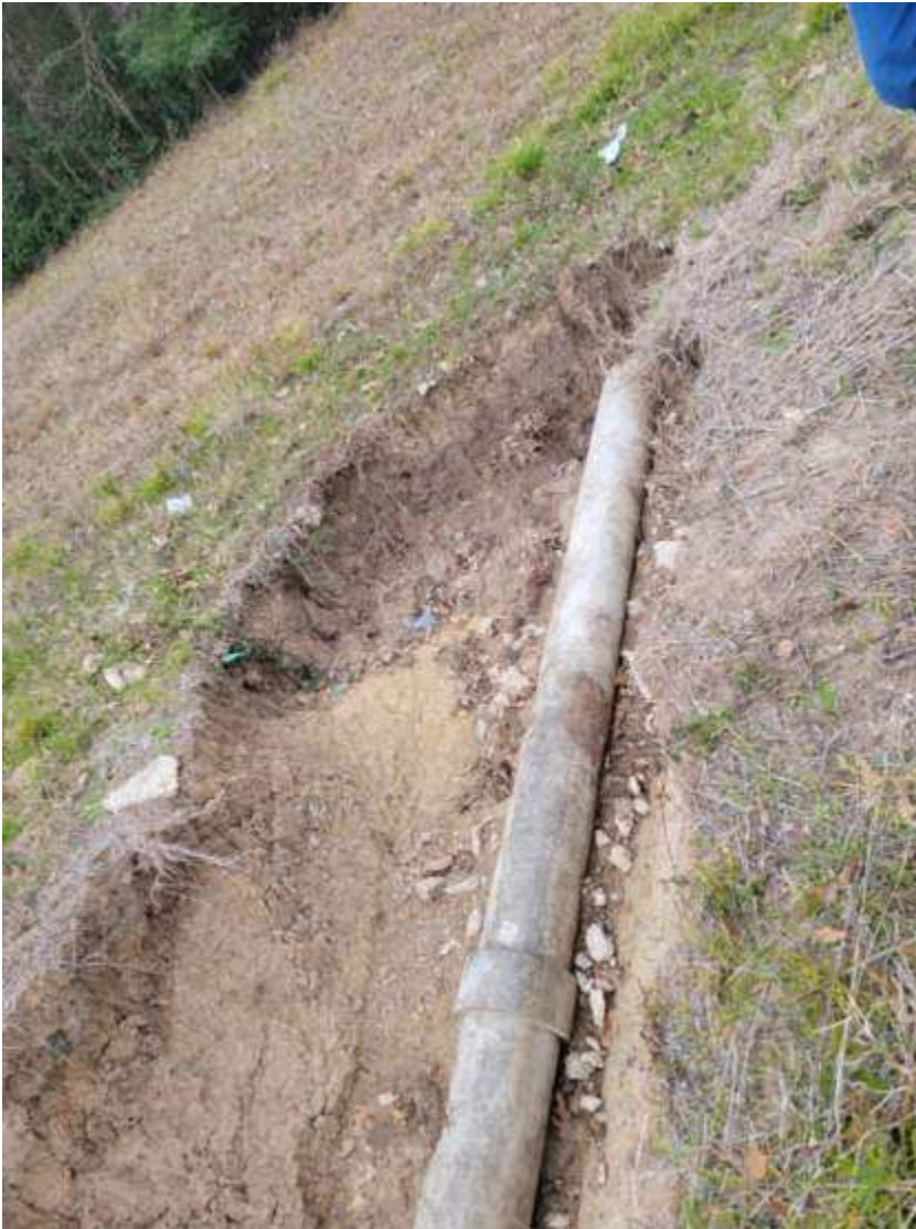
Public Works Staff found serious erosion around City's Main waterline off the Bypass
