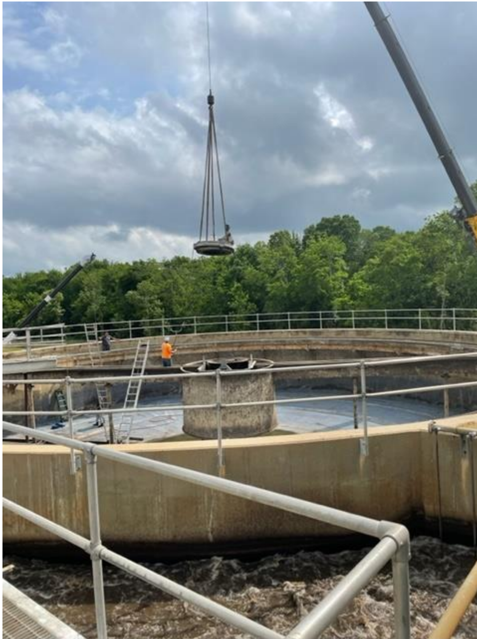
Wastewater Treatment Plant Clarifier
