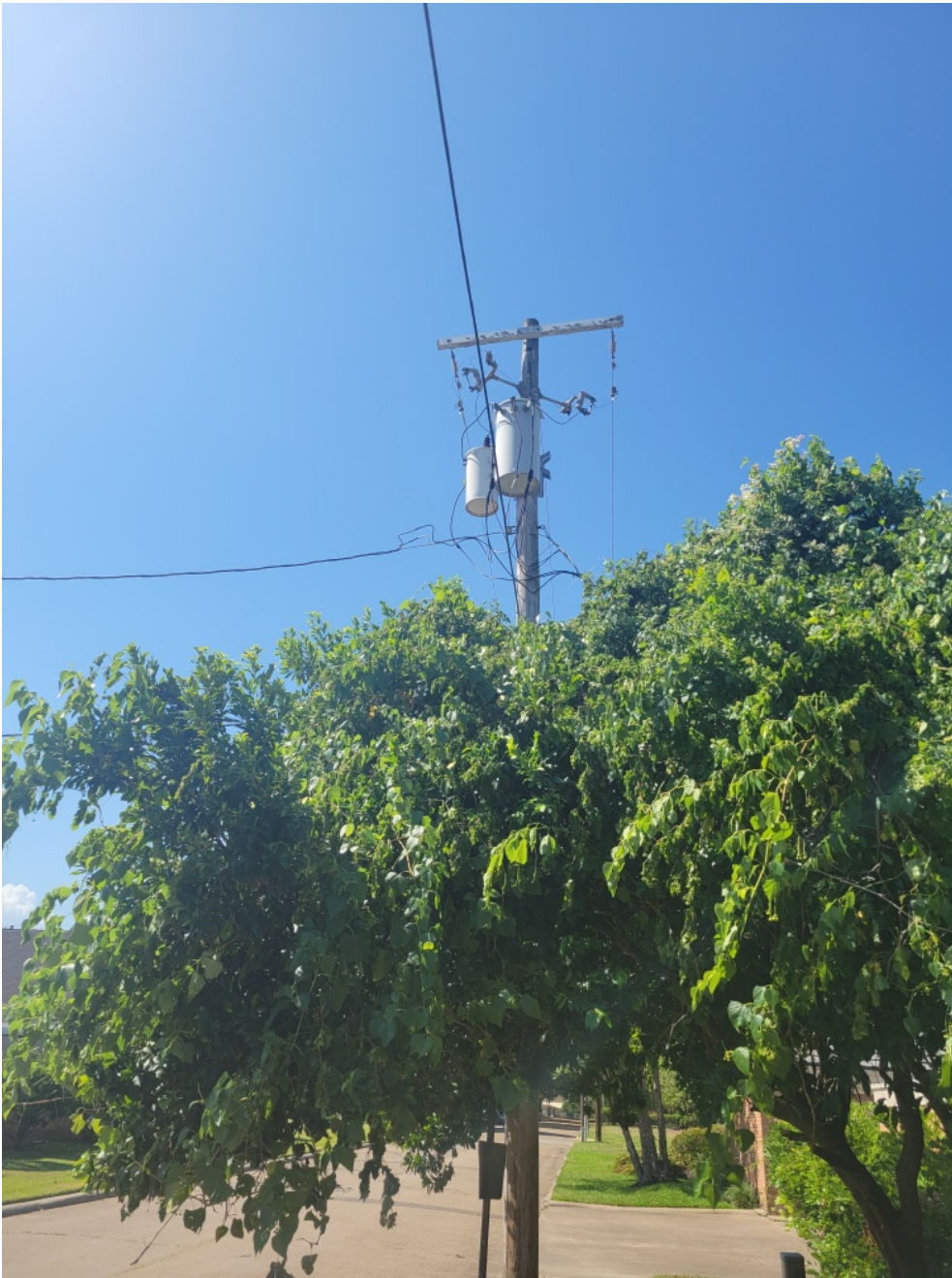
Vines removed from transformers by Texas Elite
