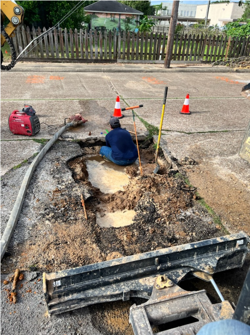
WATER LEAK ON SAM HOUSTON ST; JOEL
