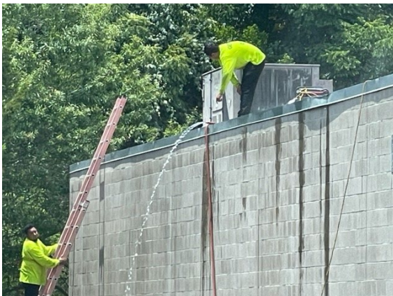
An unexpected waterline was cut into.
