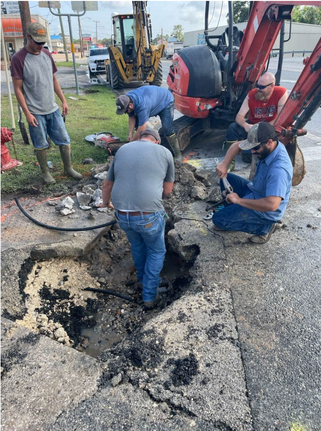
WATER LEAK ON GRAND AND MAIN
