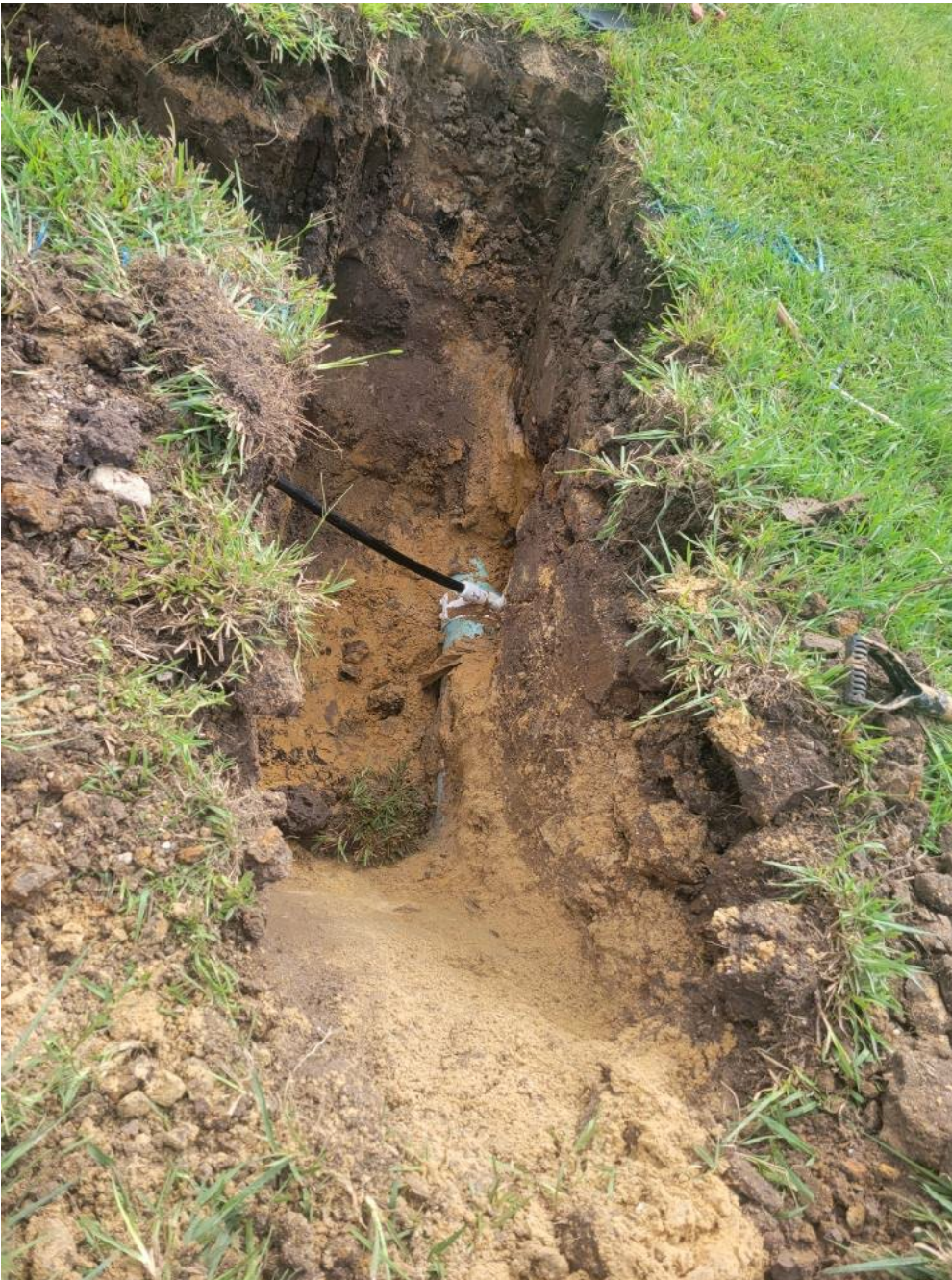
TAPPED WATERLINE ON TIMBER RIDGE
