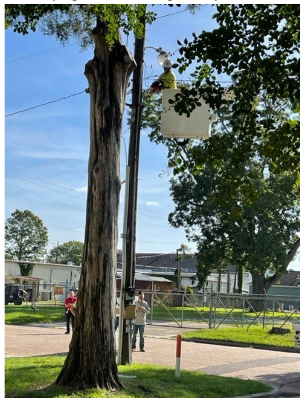
The pole that was damaged by a squirrel. Liberty Fire Dept. Captain Eric McDaniel on the left.
