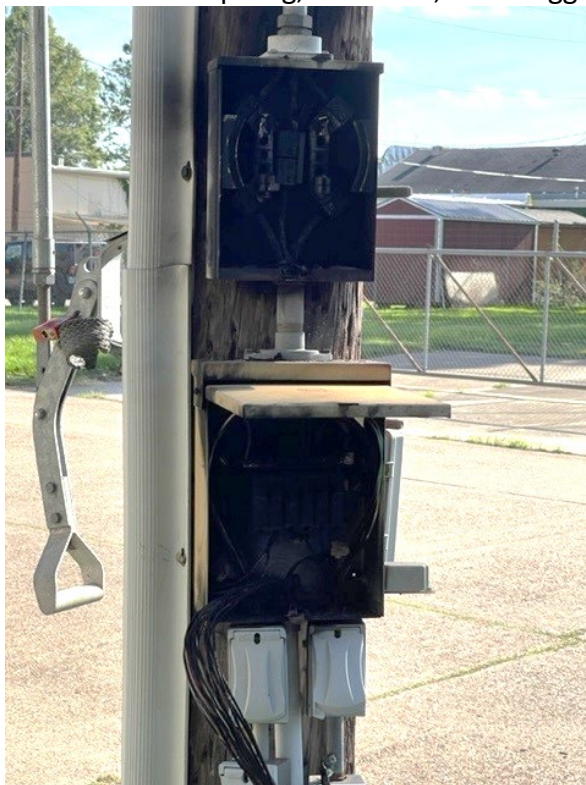
Torched electric meter and breaker box.
