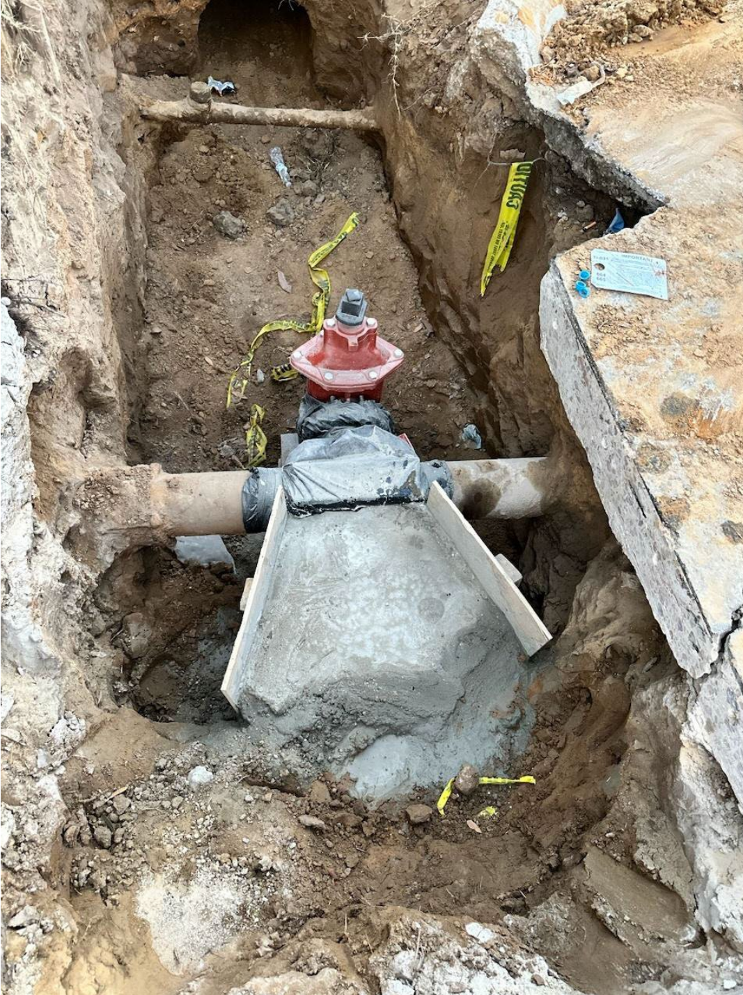
WATERLINE TAP AND VALVE ON MAPLE ST.
