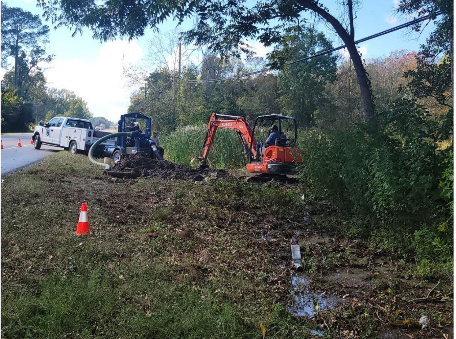
WATER LEAK ON NORTH MAIN ACROSS FROM RIDGEWOOD
