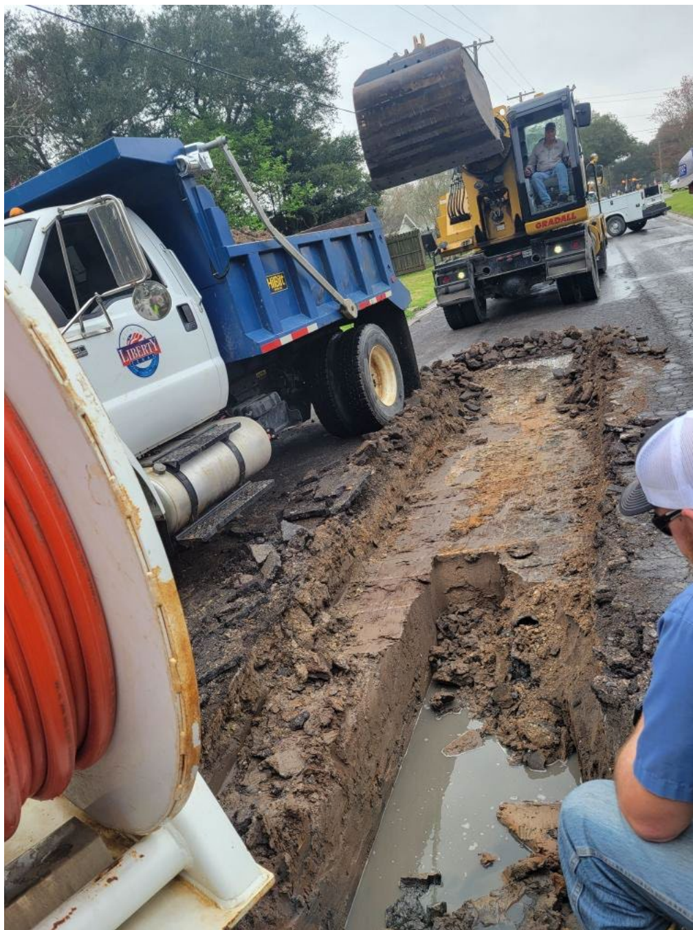
SANITARY SEWER ISSUE AT WILLOW AND NORTH TRAVIS – DAVID, AND RICK
