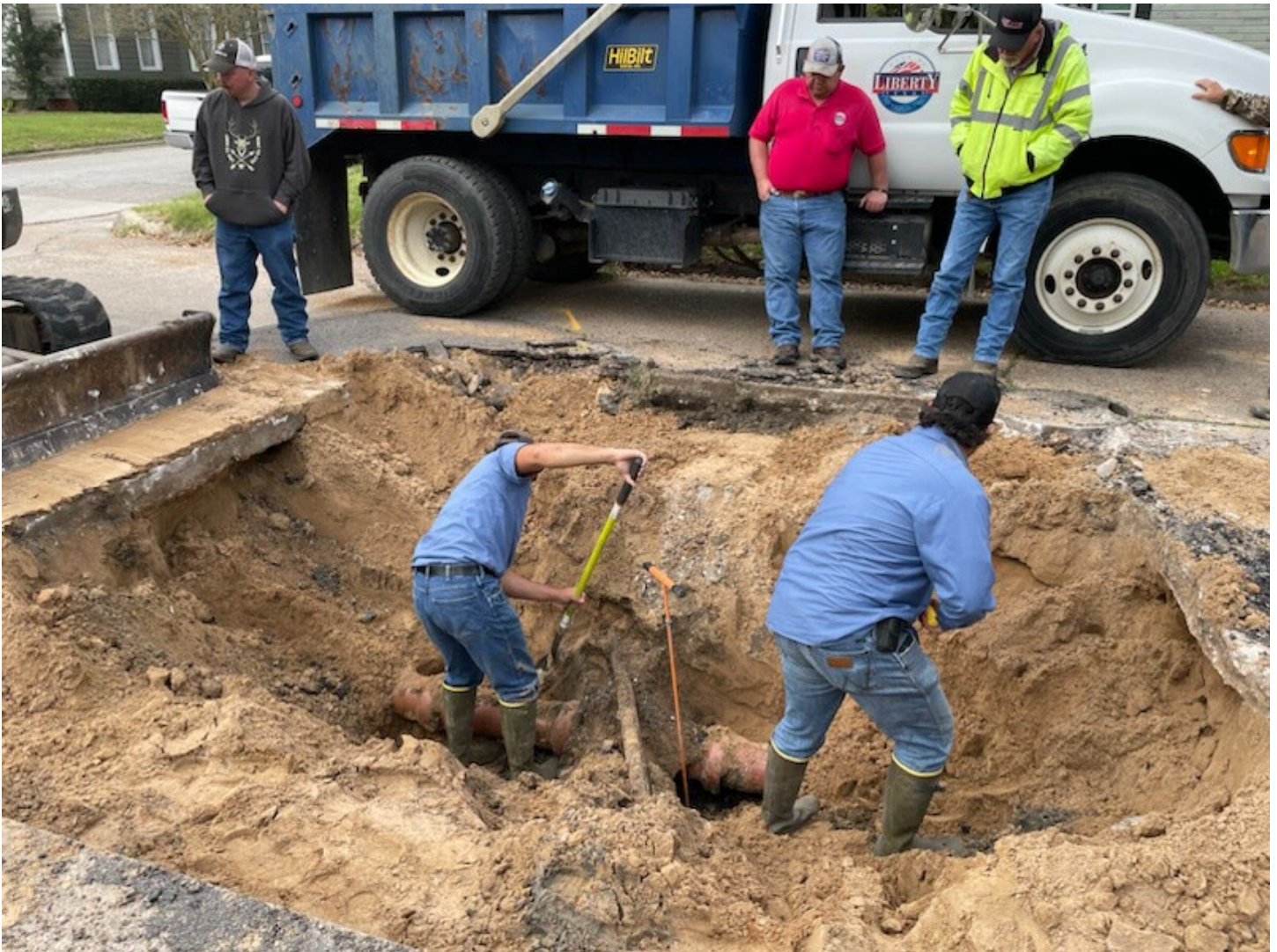
SANITARY SEWER LINE BREAK ON BOWIE – JOEL, CHRISTIAN, JAMES, RAYMOND, AND ROBERT
