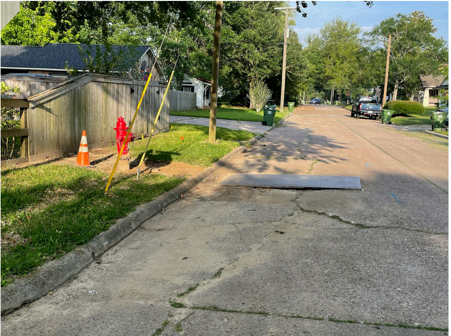
NEW FIRE HYDRANT AT KENTUCKY AND WEBSTER
