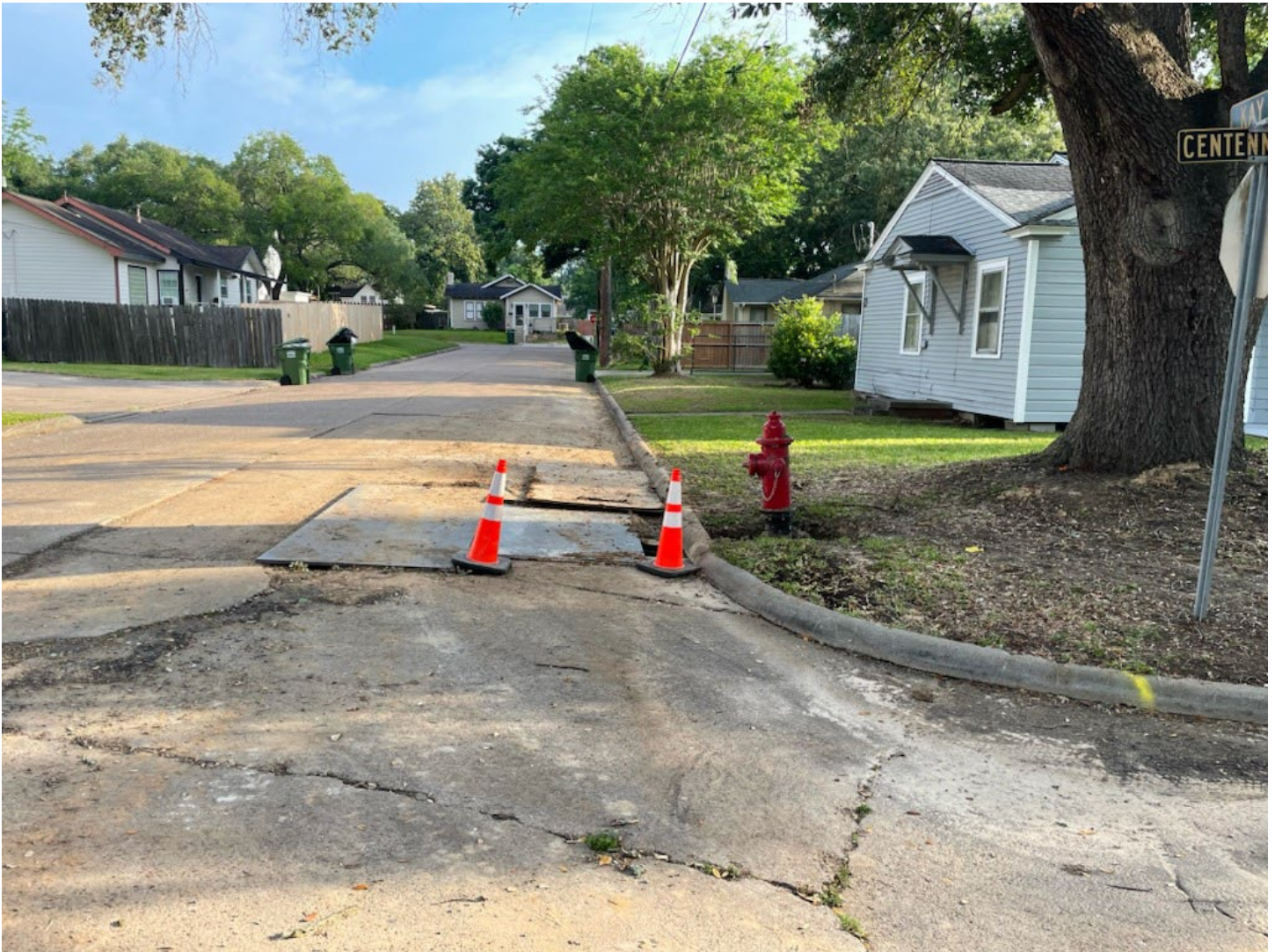
NEW FIRE HYDRANT AT KAY AND CENTENNIAL
