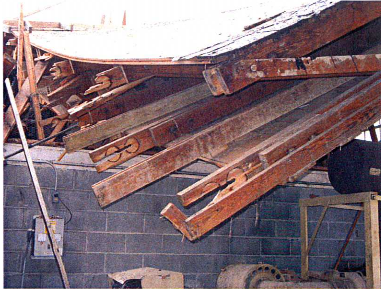
Truss End With Failed Split Ring Connector
