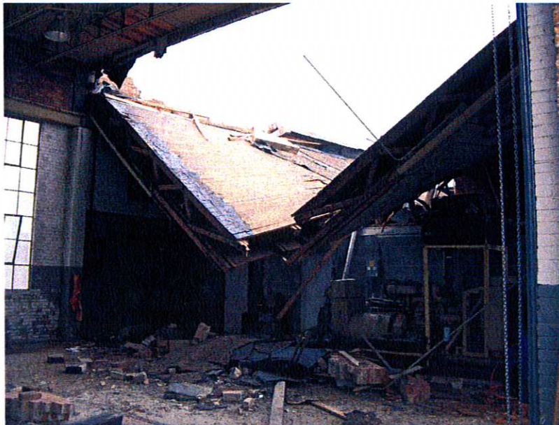
Collapsed Roof Structure
