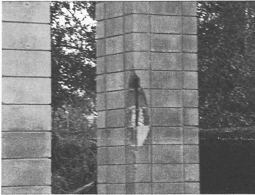
Masonry Cell without Grout
