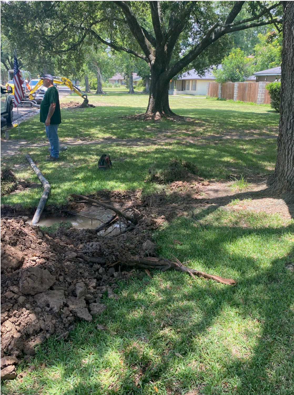
WATER LEAK CAUSE BY CENTERPOINT CONTRACTOR ON STAR RIDGE AND ATASTOCITA
