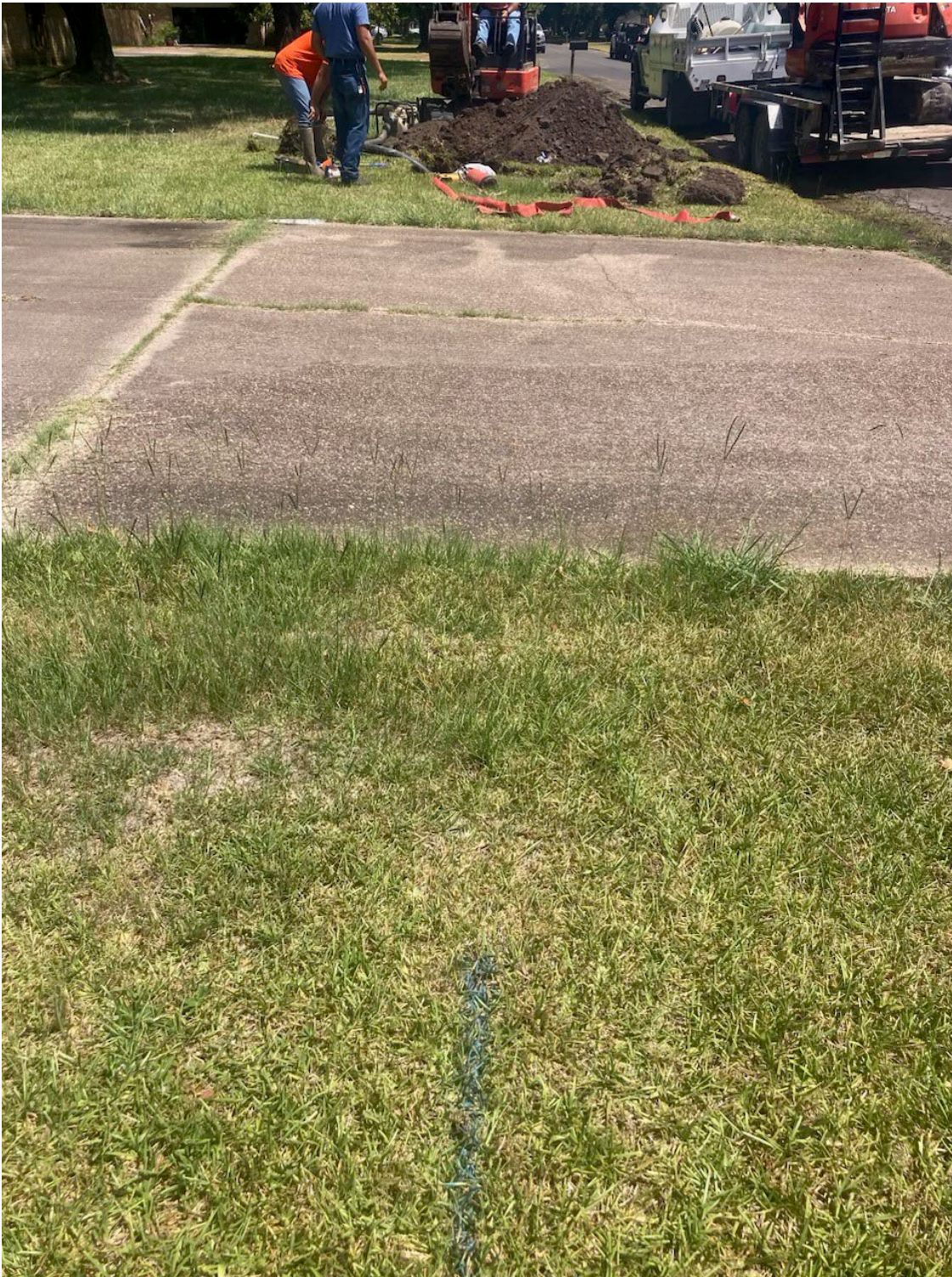
WATER LEAK CAUSED BY CENTERPOINT CONTRACTOR ON NORTH TRAVIS
