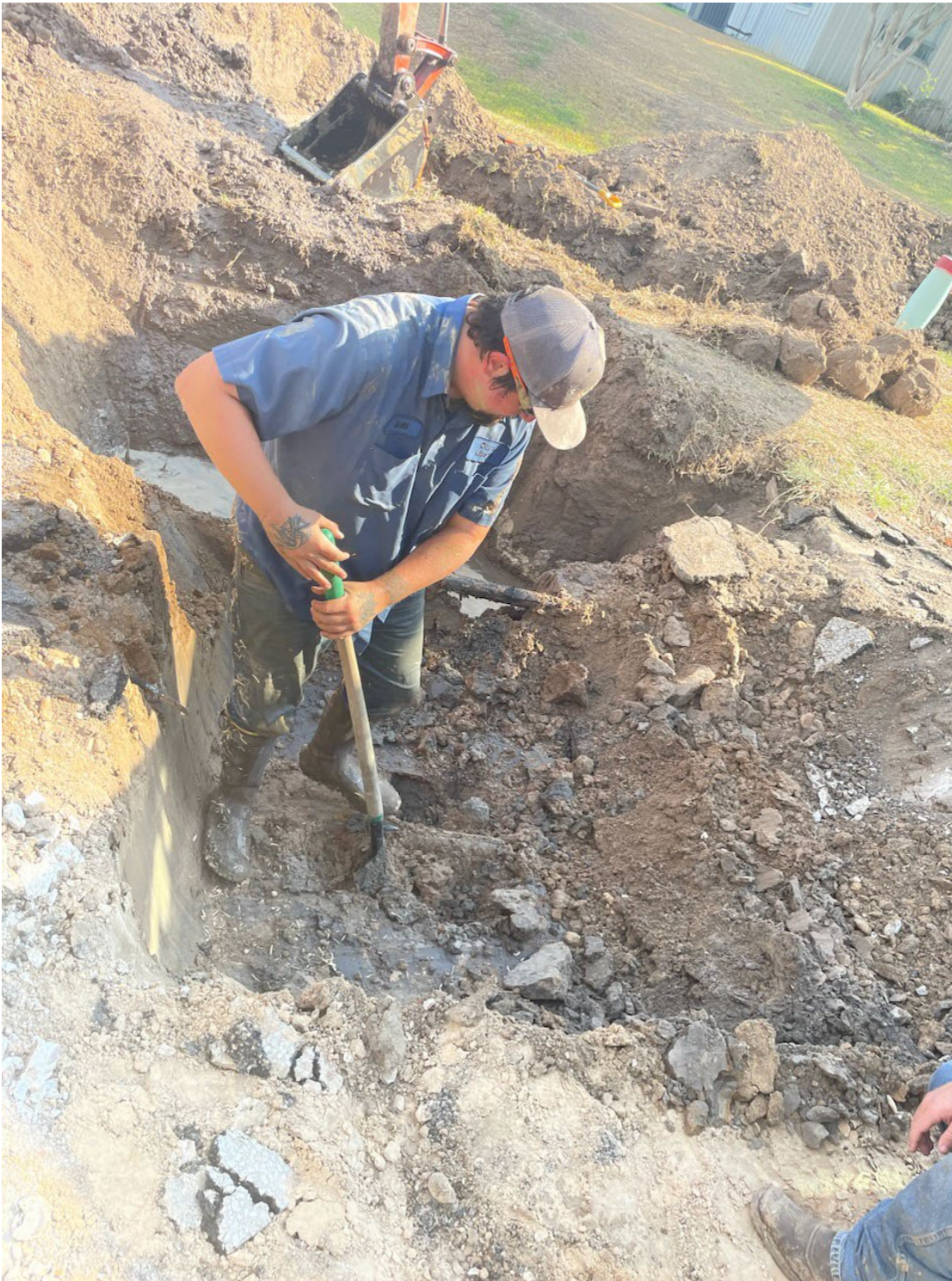
WATER LEAK ON BEAUMONT AND KENTUCKY IN THE STREET, JOEL
