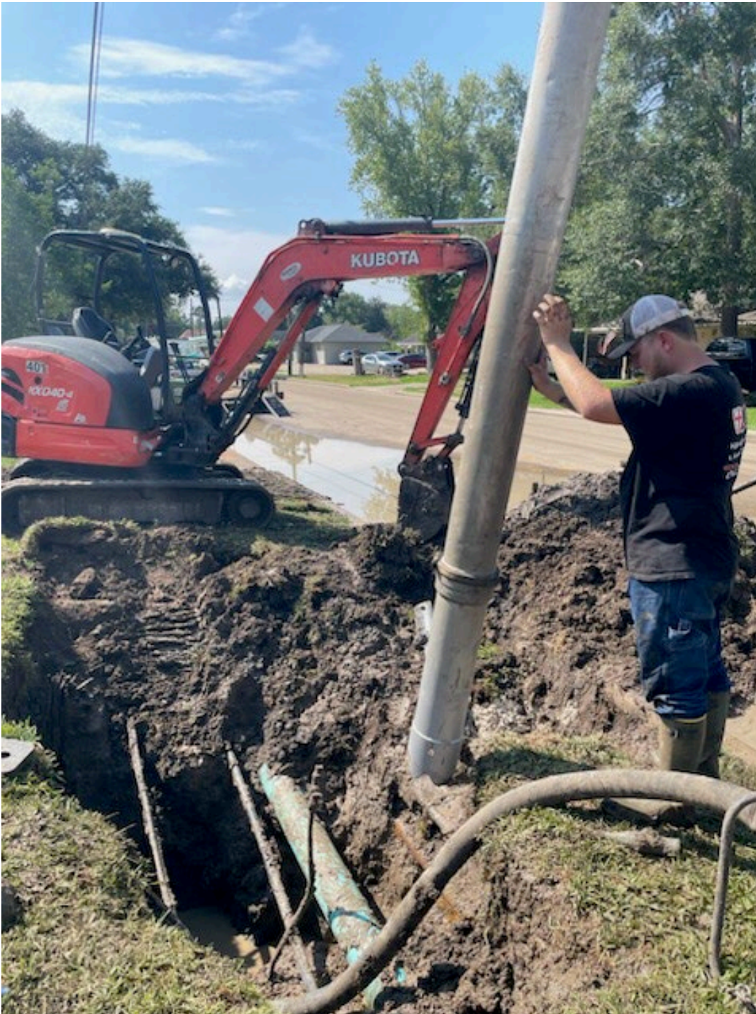
WATER LEAK ON NORTH TRAVIS
