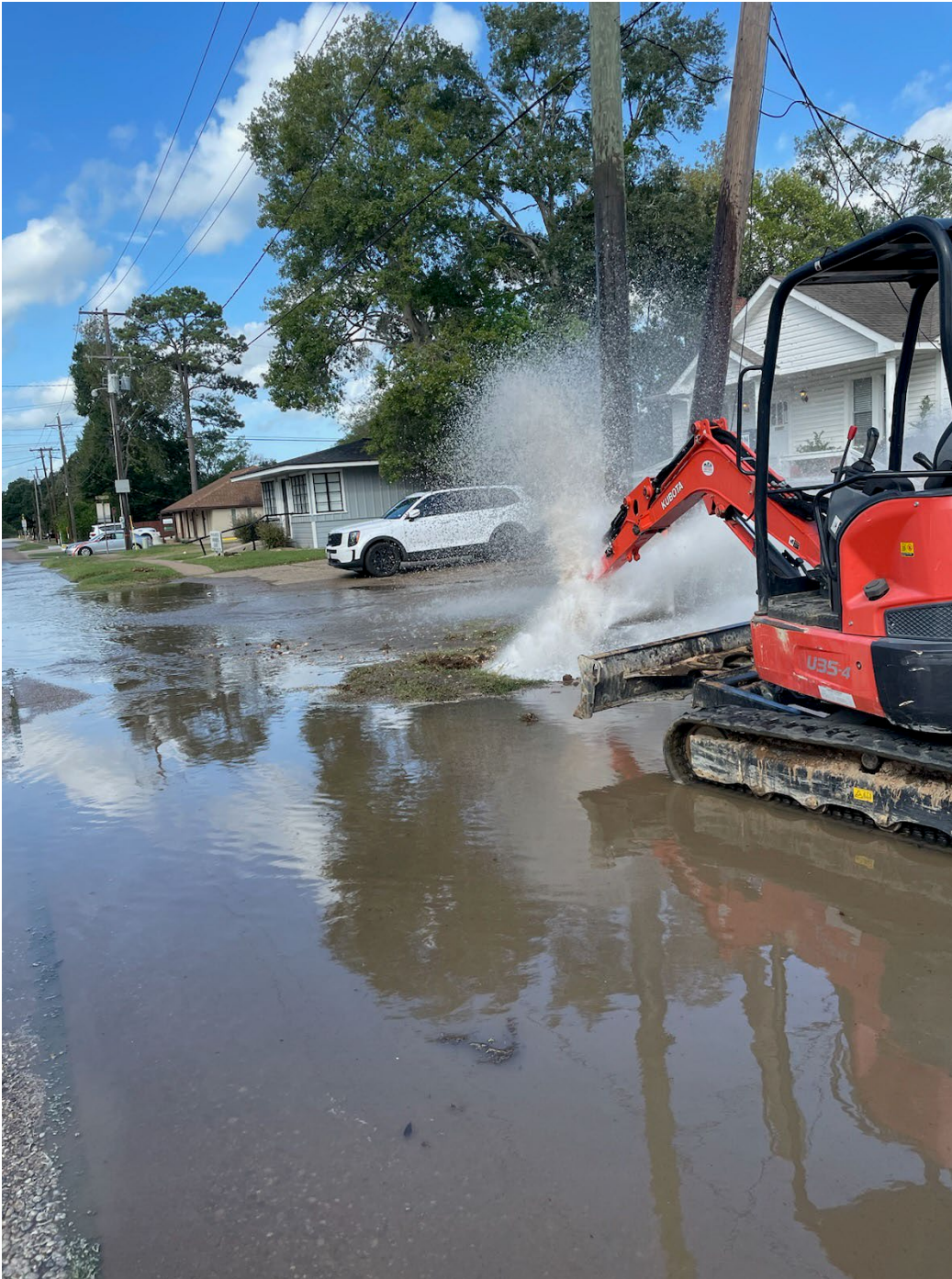
WATER LEAK AT TRAVIS AND GRAND CAUSED BY CONTRACTOR
