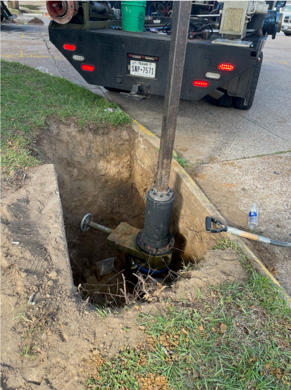
WATER LEAK AT TRAVIS AND GRAND LINE STOP INSTALLATION
