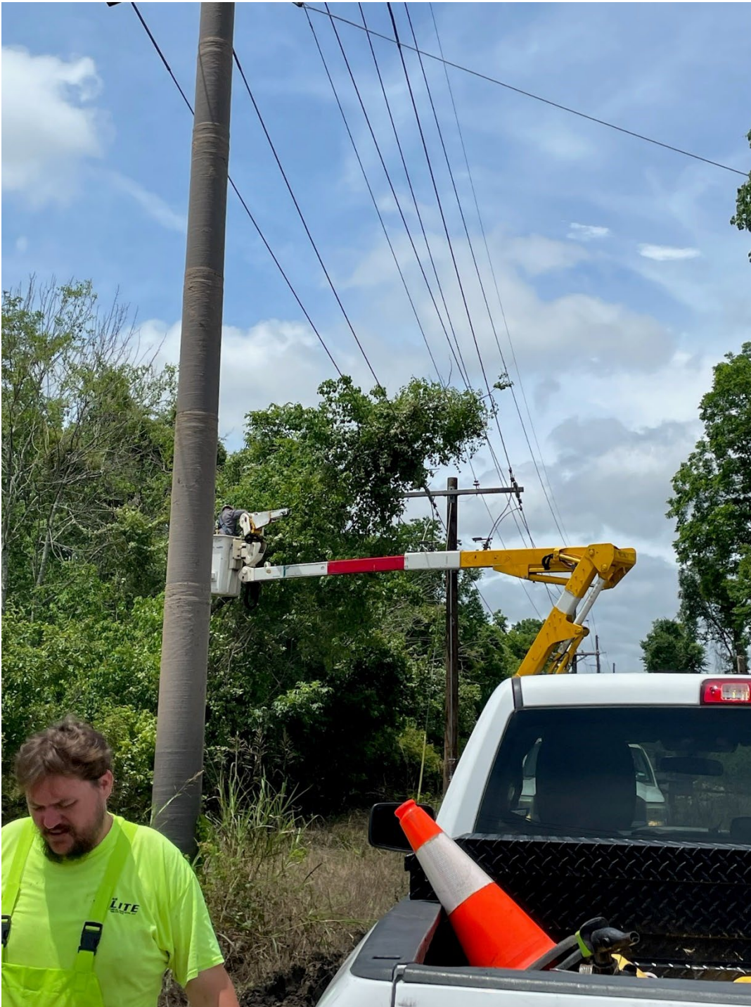
TREE OUTSIDE THE UNDEVELOPED MILAM STREET EASEMENT TRIPPED OUT LIBERTY SUBSTATION ON MAY 31. TREE IS ON PRIVATE PROPERTY
