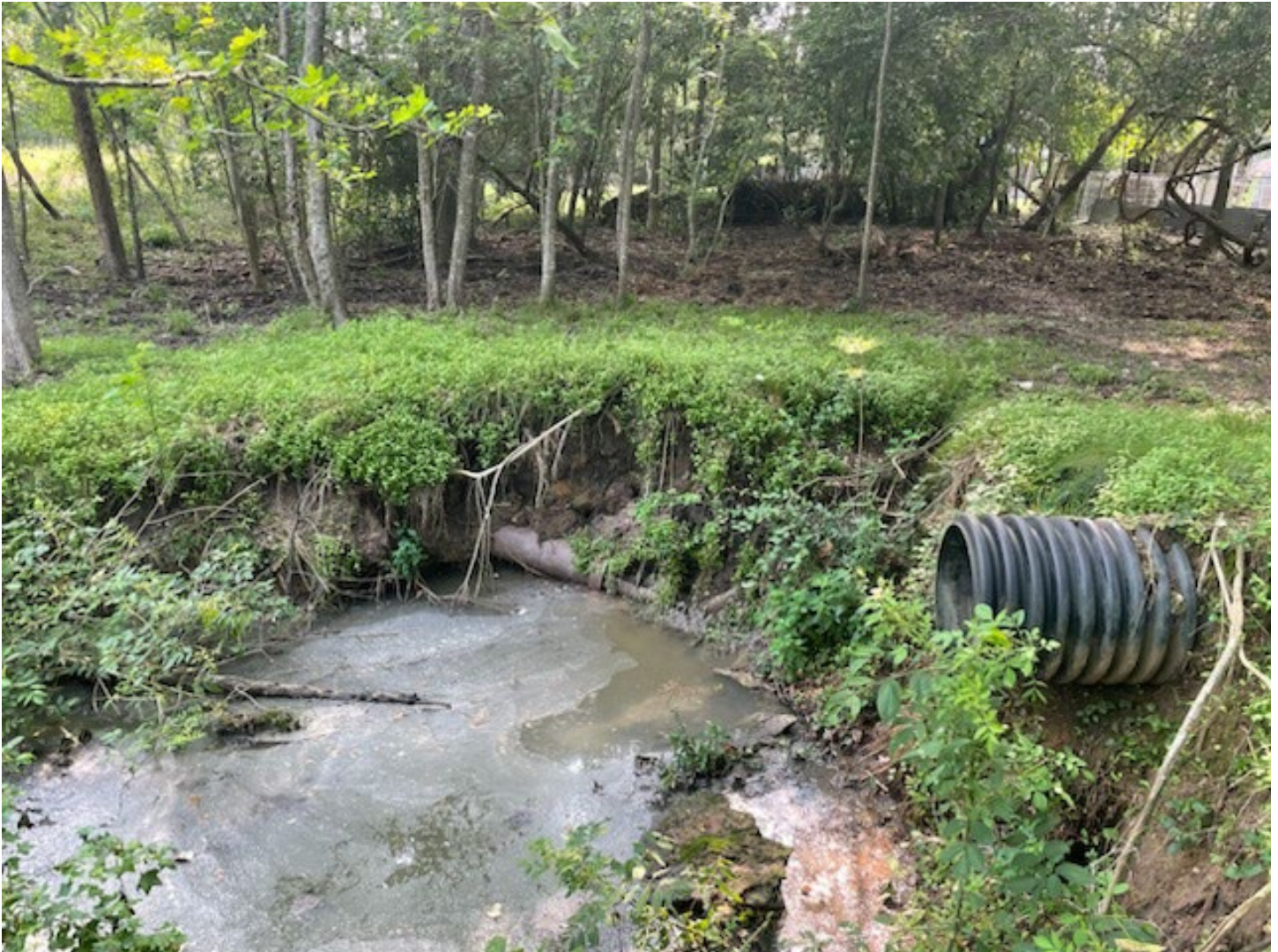
CAVITY BEHIND WILLOW ON MAIN A DITCH – EROSION
