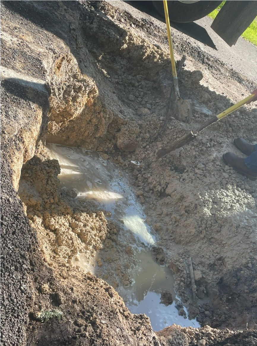
Sanitary sewer cavity on Washington St.
