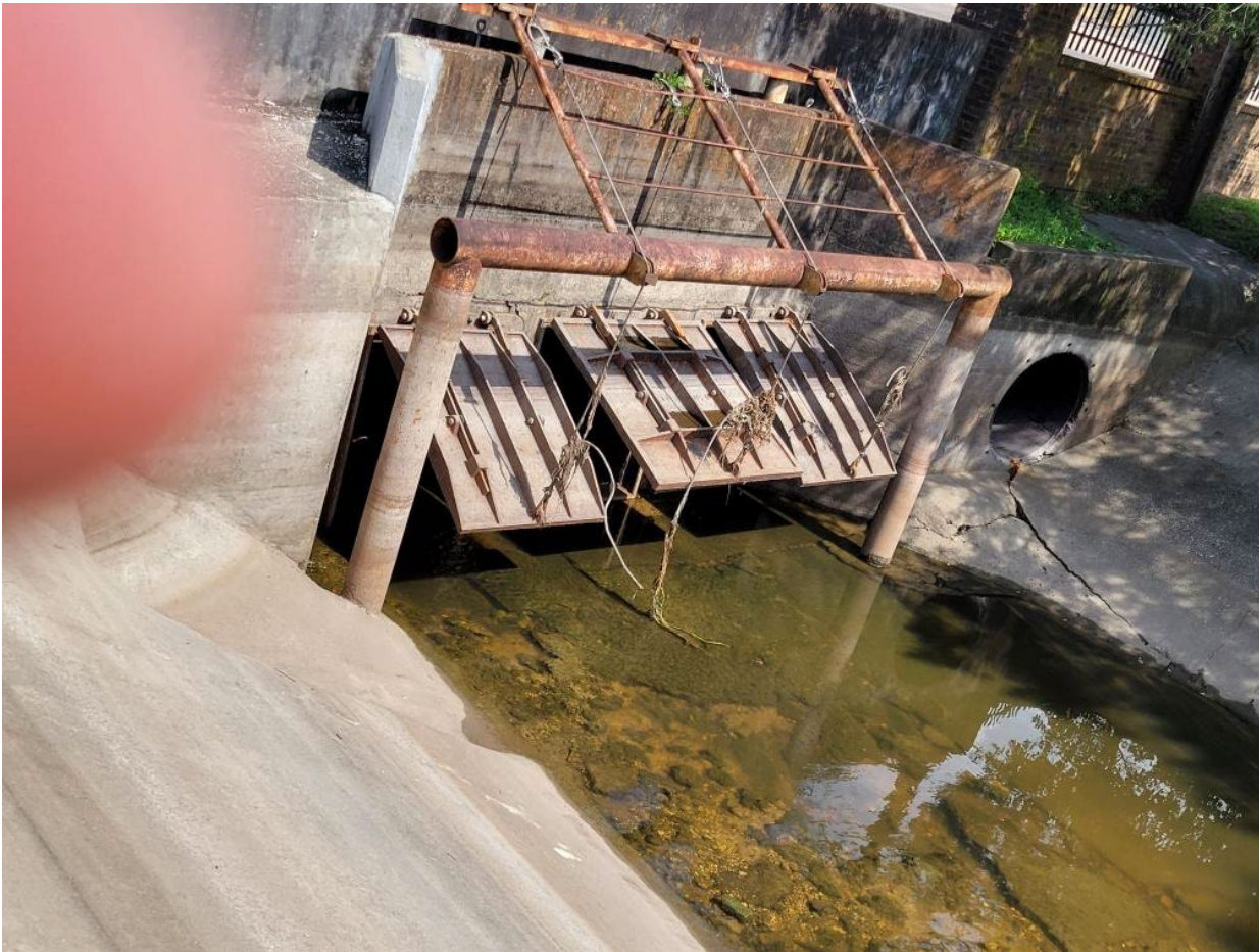
Main A & B flap gates were open on 8/6/2024.
