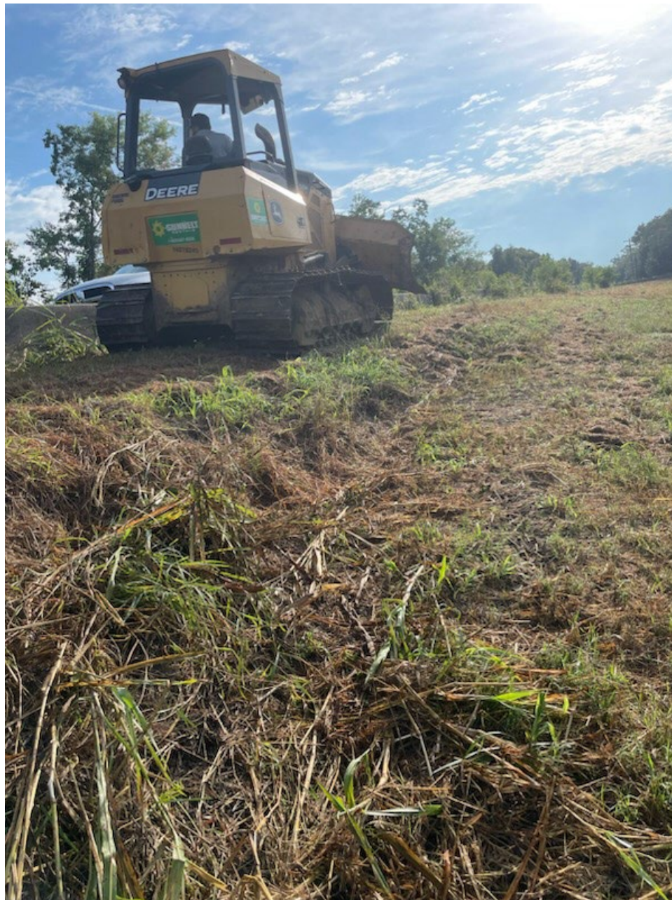
Main A Levee Failure after May 2024 Flood Event
