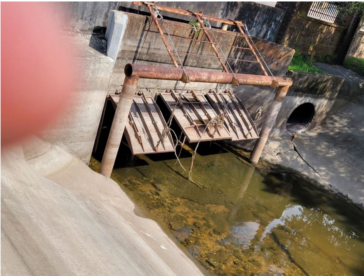
Main A & B flap gates are open
