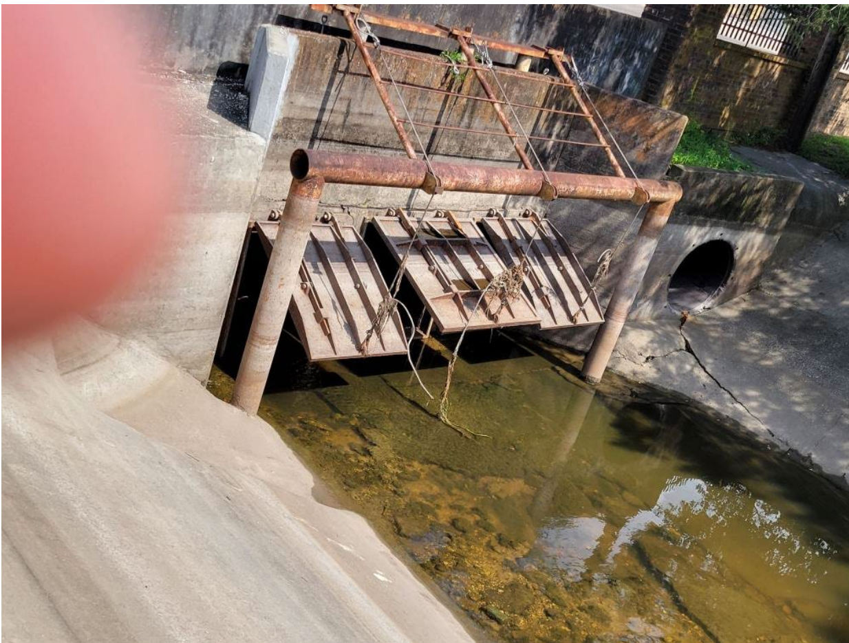
Main A & B flap gates are open
