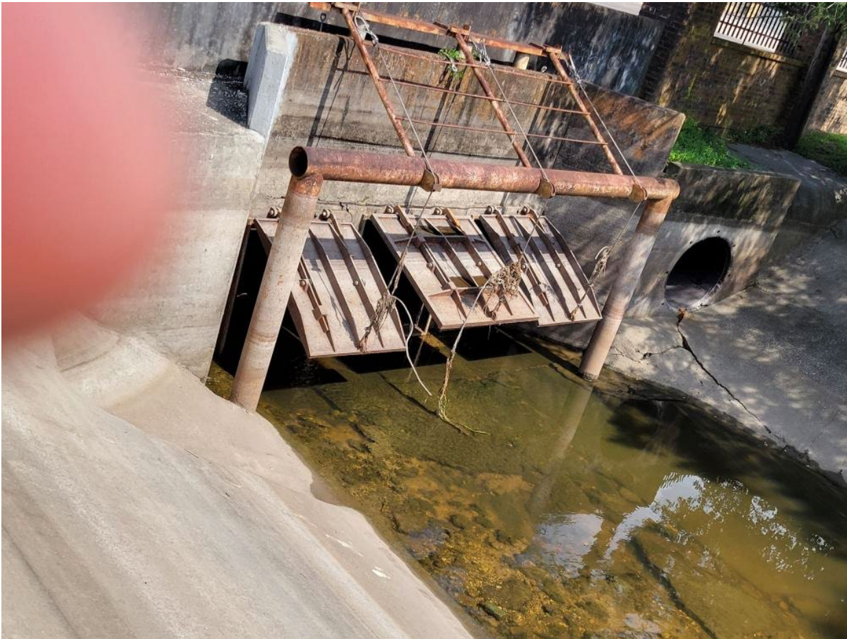
Main A & B flap gates are open
