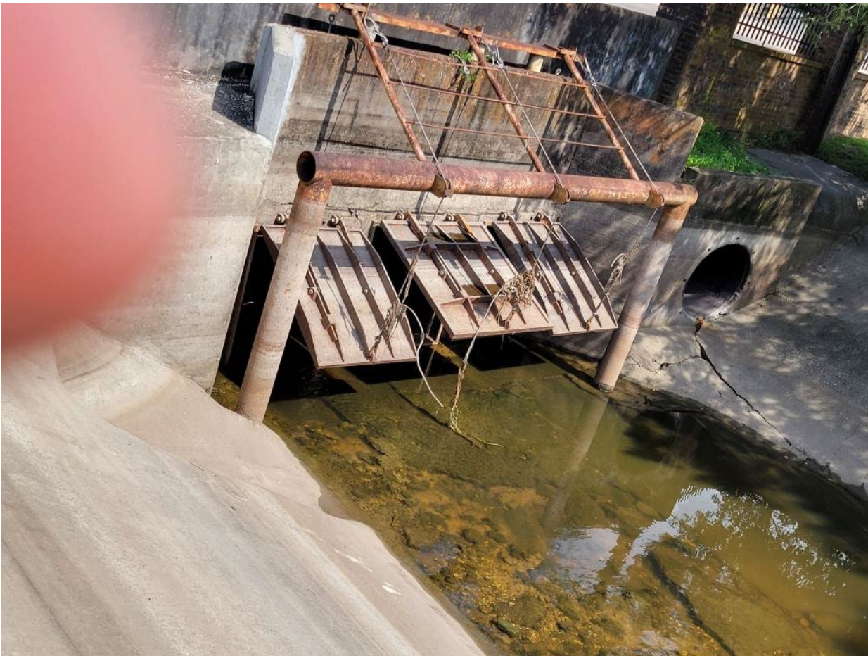
Main A & B flap gates are open
