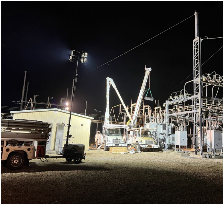
LIBERTY SUBSTATION DURING THE CITY WIDE OUTAGE ON DECEMBER 14 - 15
