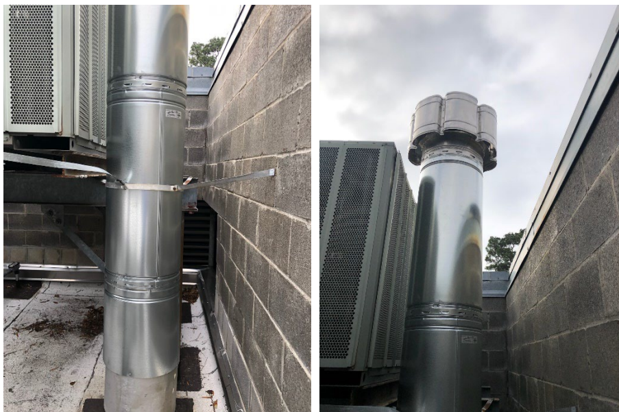
New Boiler Pipe Flue and Cover
