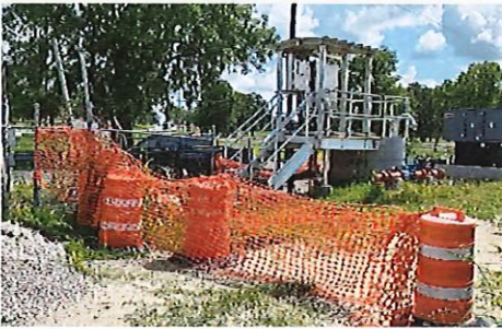
MCGUIRE LIFT STATION
