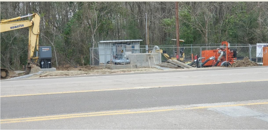
BYPASS LIFT STATION
