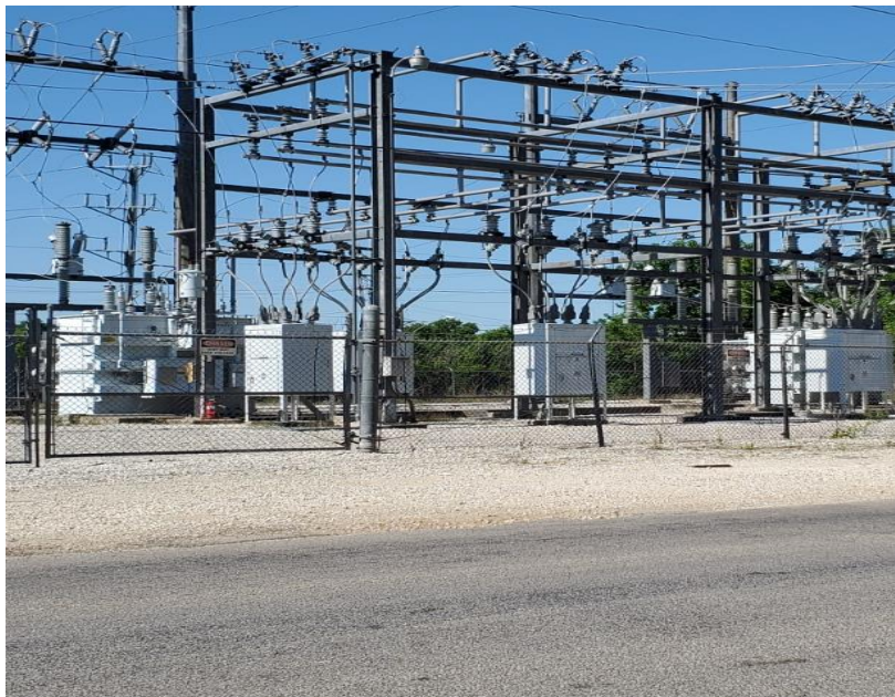
BEAUMONT ELECTRICAL SUBSTATION – ON BEAUMONT AVE.
