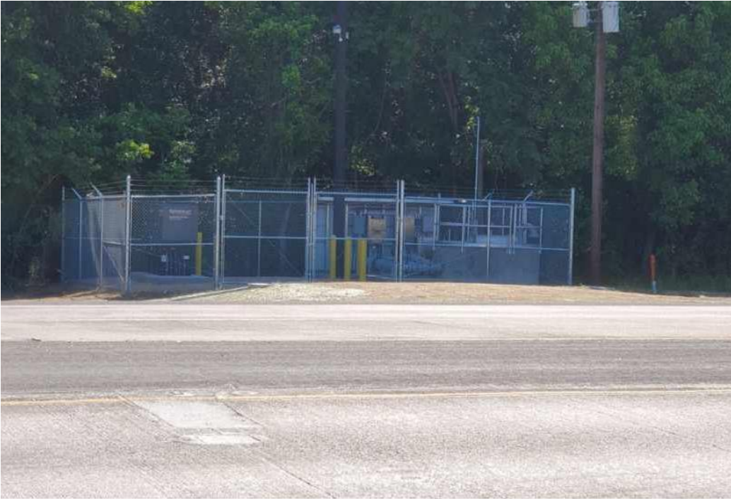
BYPASS LIFT STATION
