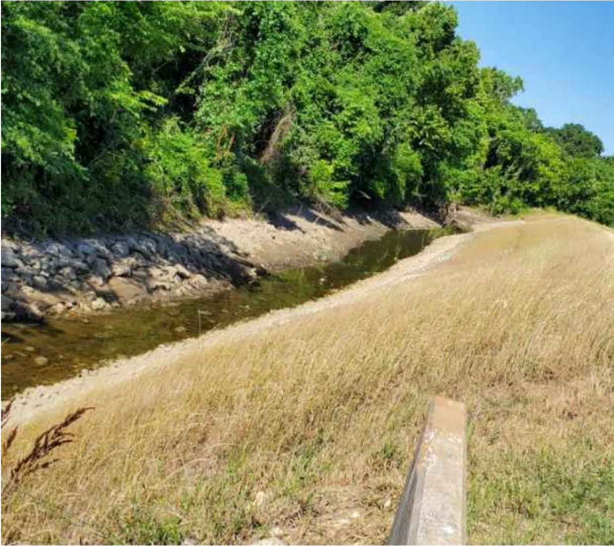
MAIN B LEVEE REPAIR – VEGETATION ON SLOPE
