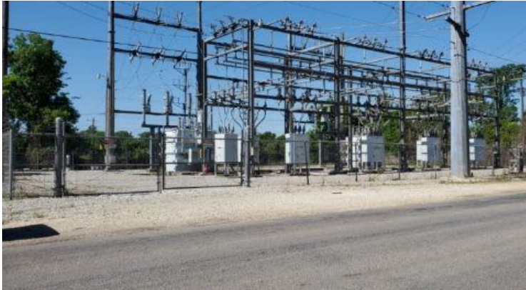
BEAUMONT ELECTRICAL SUBSTATION
