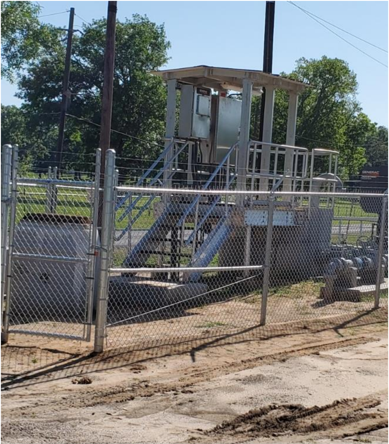
MCQUIRE LIFT STATION
