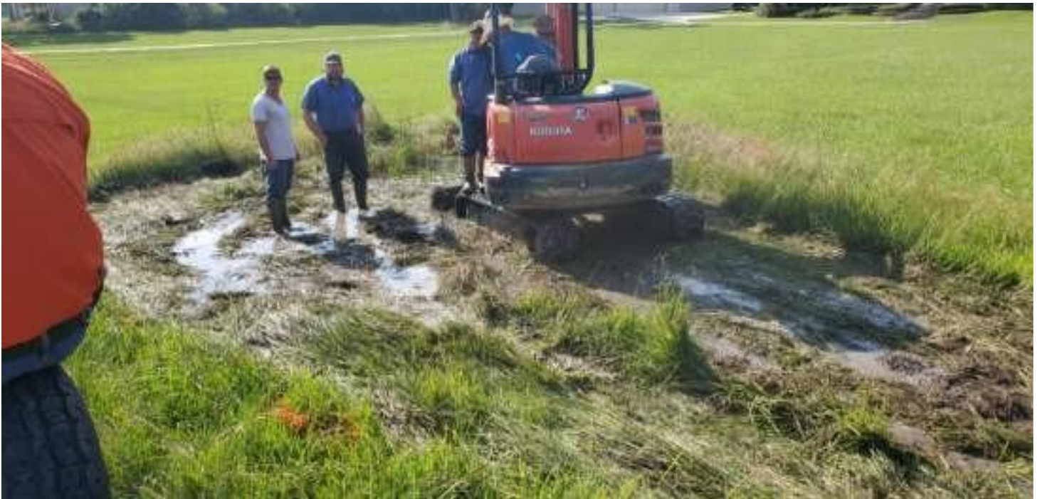
RAVENHILLS – WATER LEAK; DAVID DISKELL, JAYMES YOUNG, DAVID ALLISON AND MIKE FLINN
