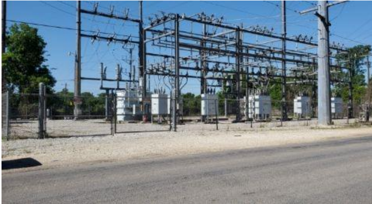
BEAUMONT ELECTRICAL SUBSTATION
