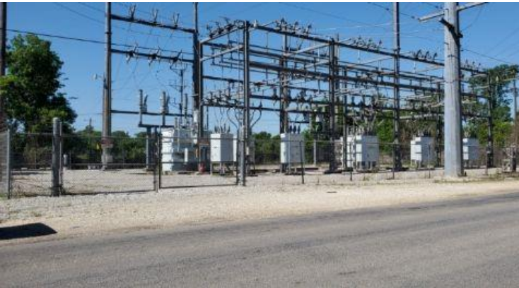
BEAUMONT ELECTRICAL SUBSTATION
