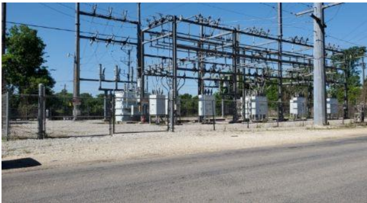
BEAUMONT ELECTRICAL SUBSTATION
