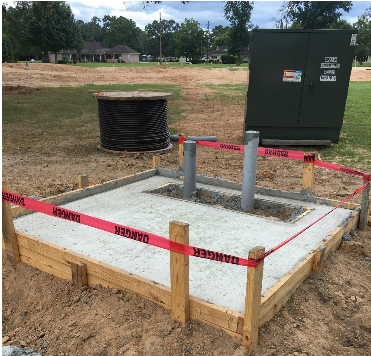
New transformer pad
