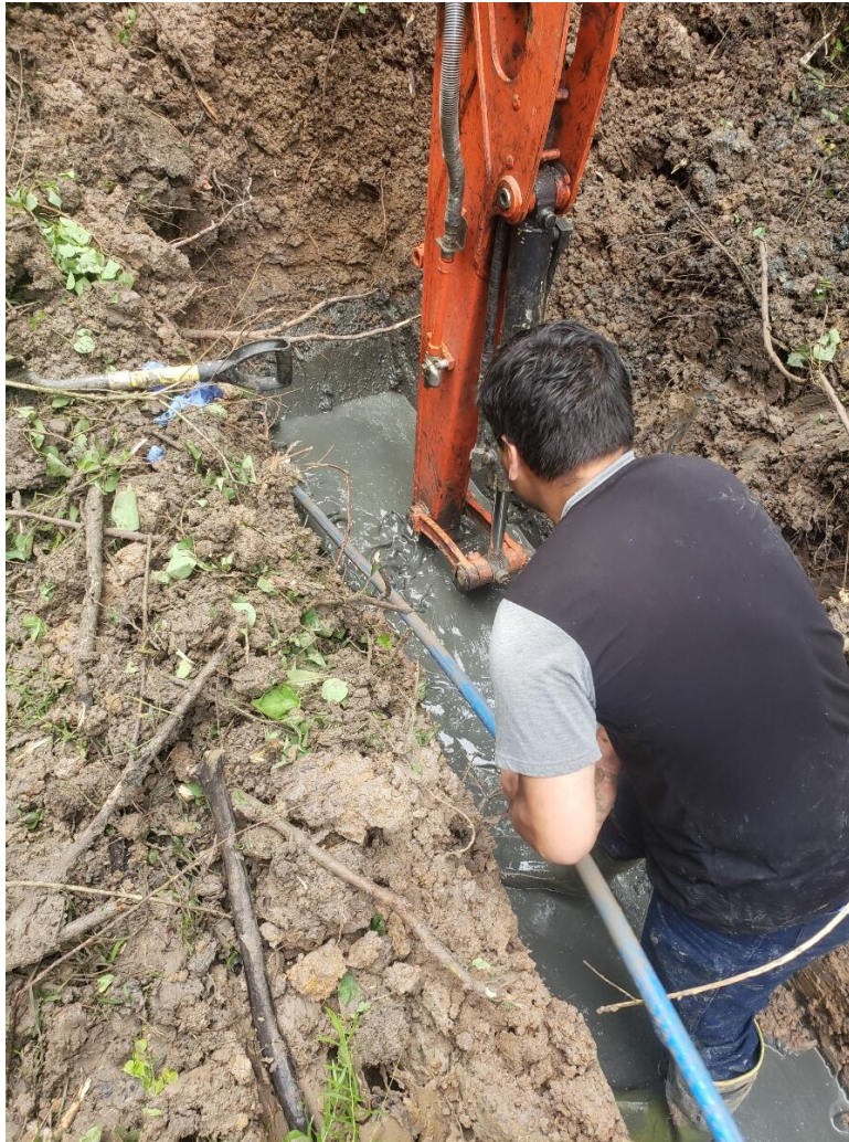
Sewer line blockage on Beaumont Ave.: Stephen
