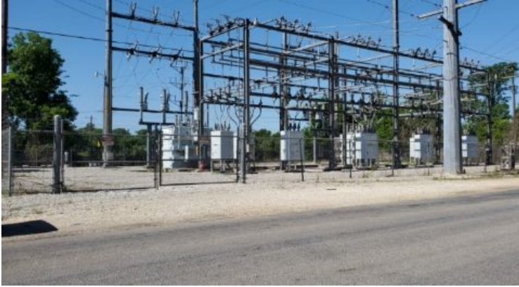
BEAUMONT ELECTRICAL SUBSTATION
