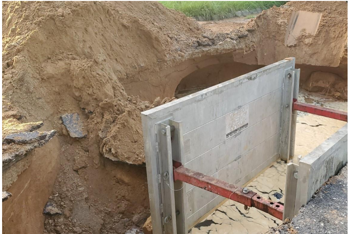
FLASHBACK: CHALLENGING CAVITY ON TEXAS ST AT HOLLY ST. NOVEMBER 2019
