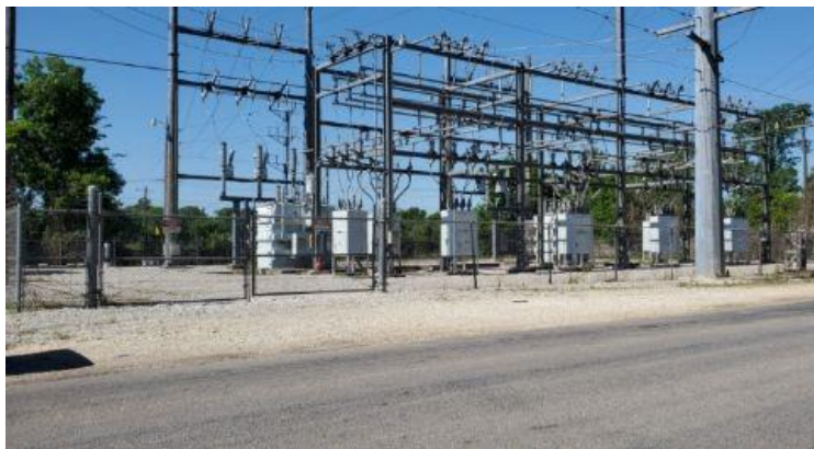
BEAUMONT ELECTRICAL SUBSTATION
