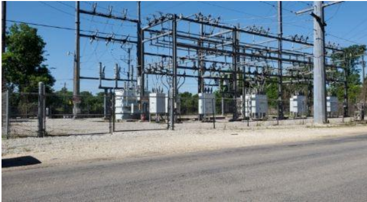
BEAUMONT ELECTRICAL SUBSTATION
