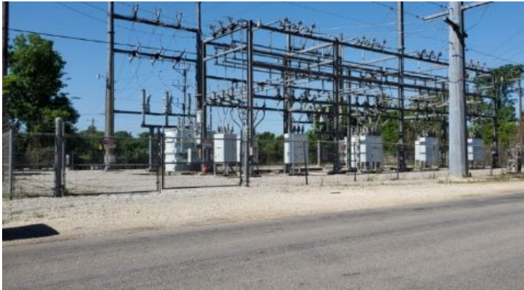
BEAUMONT ELECTRICAL SUBSTATION
