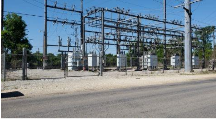
BEAUMONT ELECTRICAL SUBSTATION
